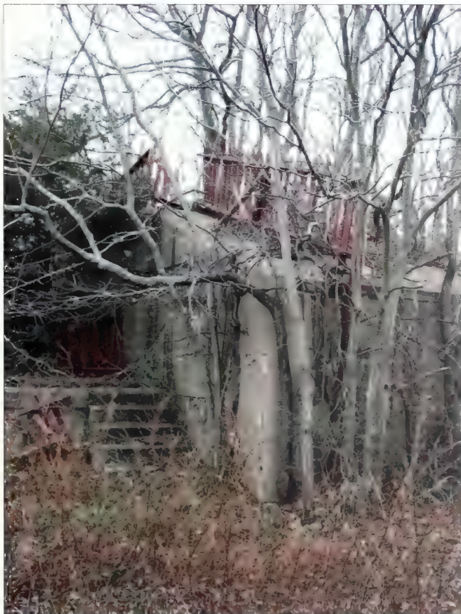
Figure 5.30. View looking northeast at Battery Morris. This image shows dense stands of hackberry ( Celtis occidentalis ) growing directly along the south face of the concrete structure (Olmsted Center, January 2009).
